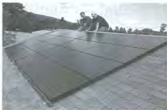
Cabot School solar panels
