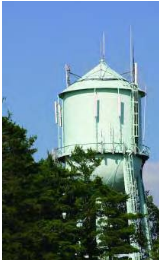
Figure 4.2: Co-locating Transmitters. Co-locating several transmitters on this water tower reduces the visual impact of multiple antenna, guy wires, and other equipment.
